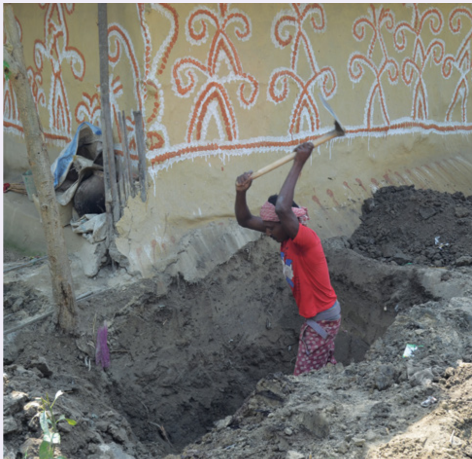
A Mushar community member digging a pit for constructing toilet. Photo credit: SDRC
