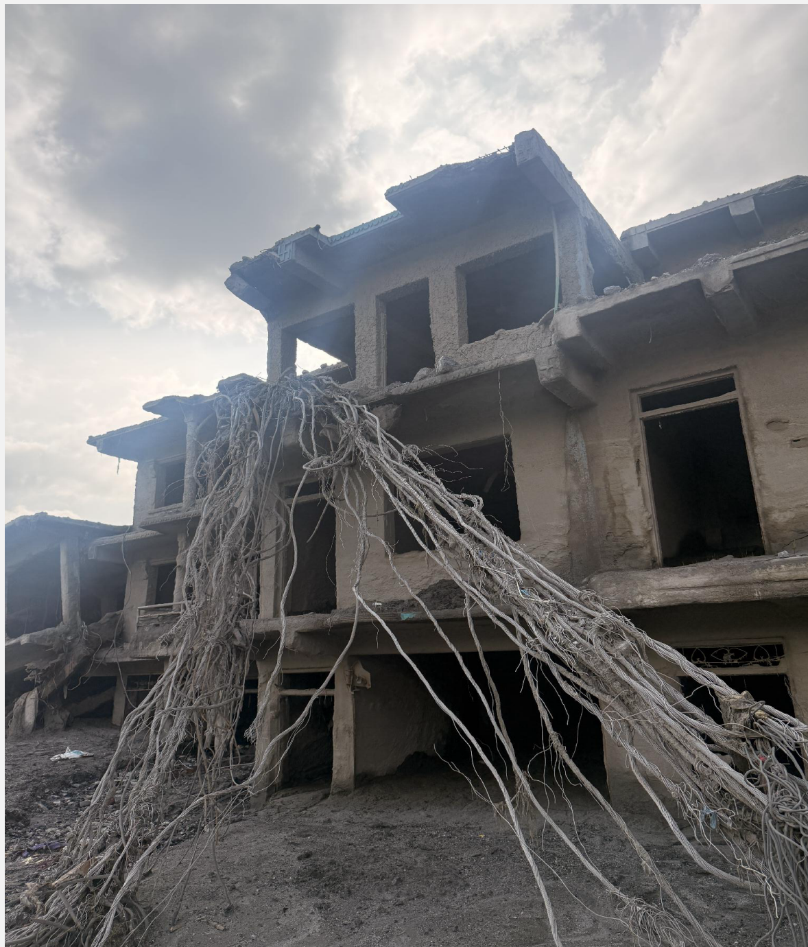
A house in Devighat destroyed by the floods. Photo: Bibhor Kayastha/Aria Technologies.
