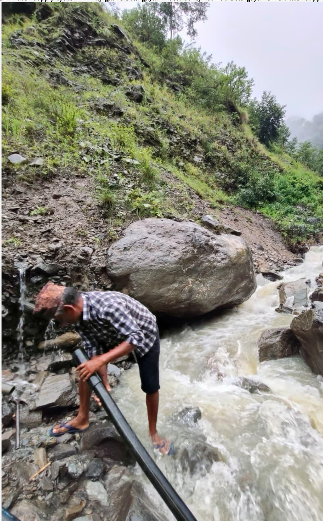
A damaged Water Supply system in Majhgaun, Uttargaya. Photo: Suraj Poudel, Uttargaya Palika water supply engineer.
