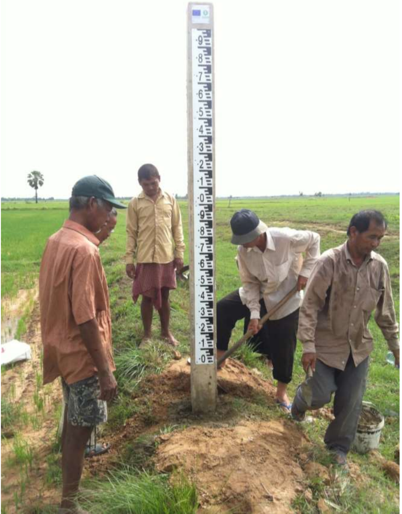
Water gauge installation in Kampong Thom province. Photo by: Oxfam
