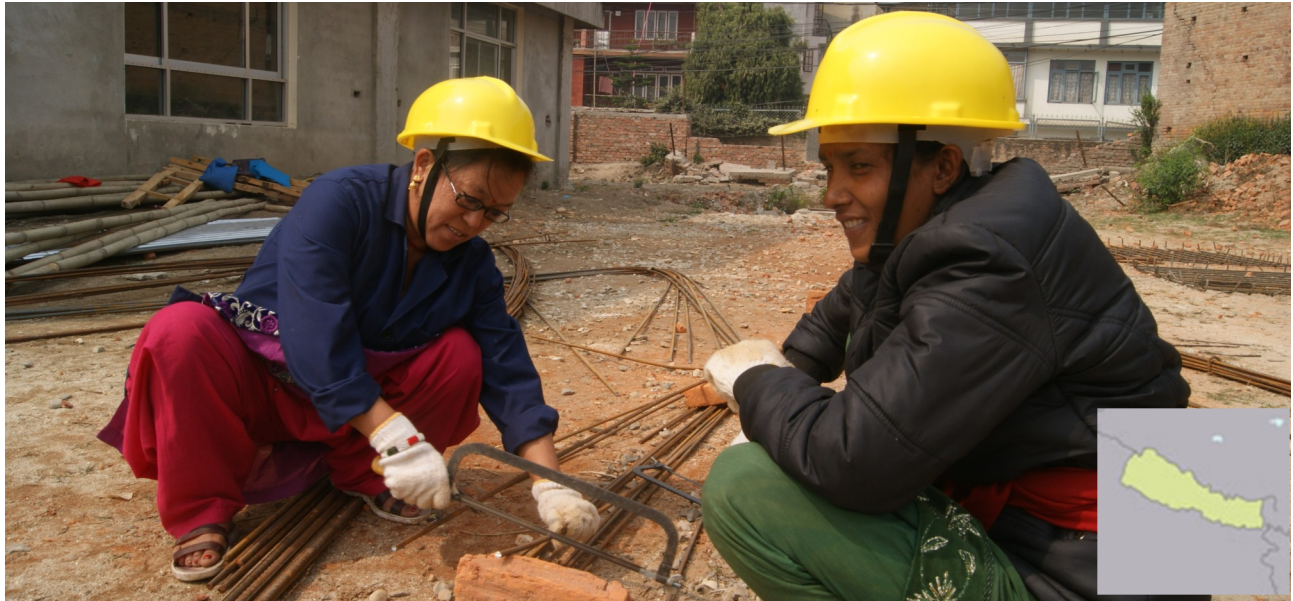
Ensuring safe shelter: women during a weeklong skilled mason training given by Oxfam and its partners on the construction of earthquake-resistant buildings in Balaju, Kathmandu on March 25, 2016. A total of 21 women participated in the training, which took place from March 22-28, 2016. Photo: Bed Prasad Dhakal/Oxfam in Nepal.
