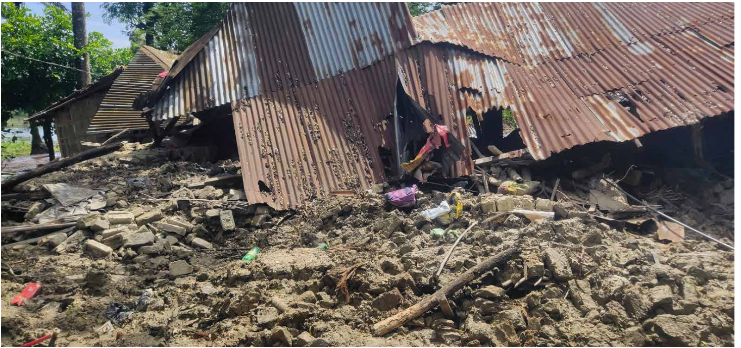
Figure 10: Flood destroyed house at Ilsaha Village in Banskhal
