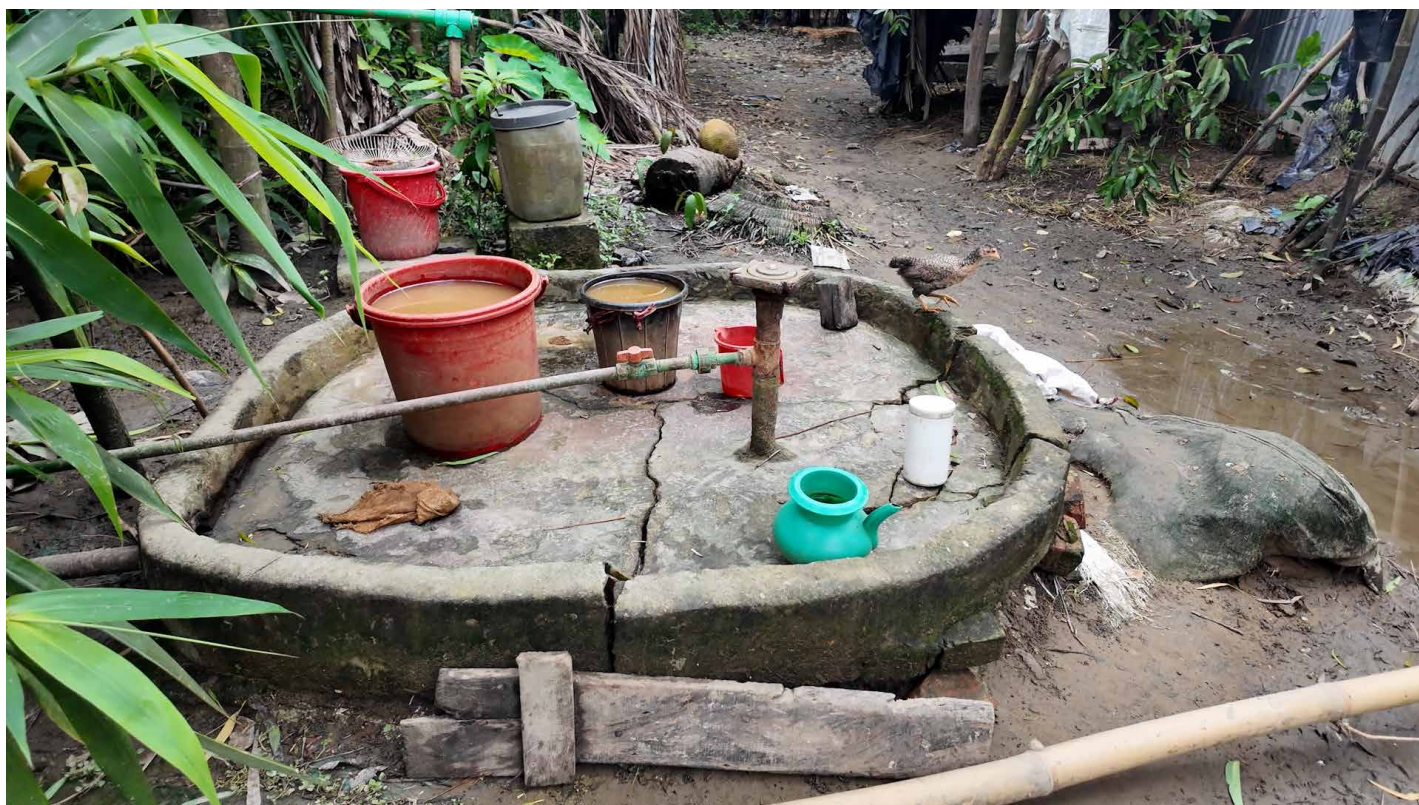
Photo: Flood-damaged tube well affecting access to safe drinking water in Satkania Upazila, Chattogram
