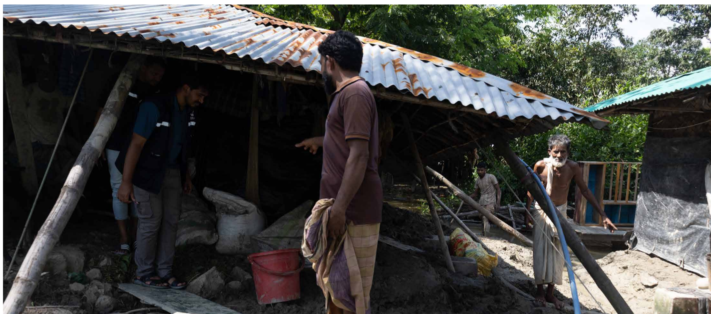
Photo: Flood-Damaged House in Ilsha Union, Banshkhali, Chattogram Photo Credit : Khondaker Mohammad Shamerul Huda, Oxfam in Bangladesh
